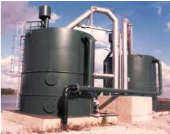
Food Industry UK Final Effluent Filtration Prior to Discharge to River 2 Single Beds Combined flow 320 m 3 /hr
