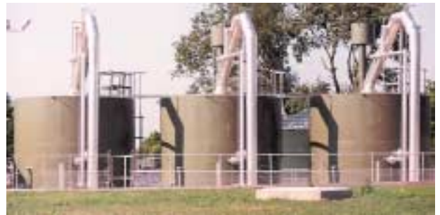
Municipal STW UK Tertiary Treatment Before Discharge to River 3 Single Beds Combined Flow 480 m 3 /hr
