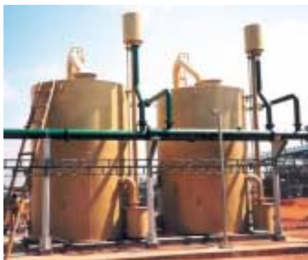
Gold Mine Mali River Water Filtration for Process 2 Single Beds Combined flow 120 m 3 /hr
