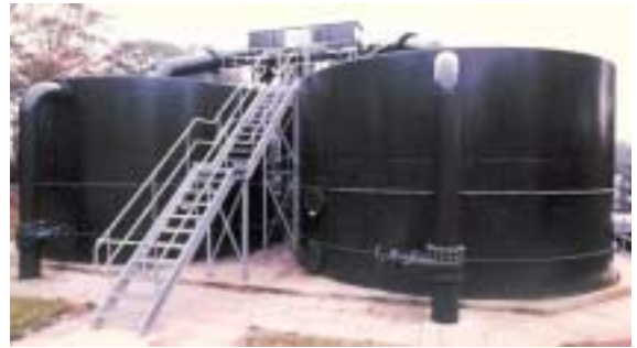
Municipal WTW UK Drinking Water Iron and Manganese Removal 2 Single Beds Combined Flow 890 m 3 /hr
