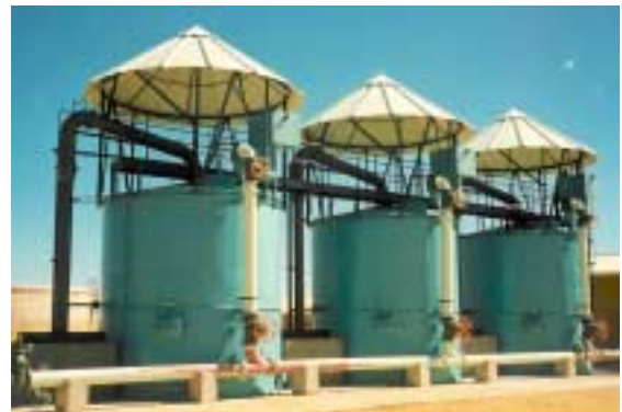
Municipal WTW Namibia River Water Filtration for Drinking 3 Single Beds Combined flow 420 m 3 /hr
