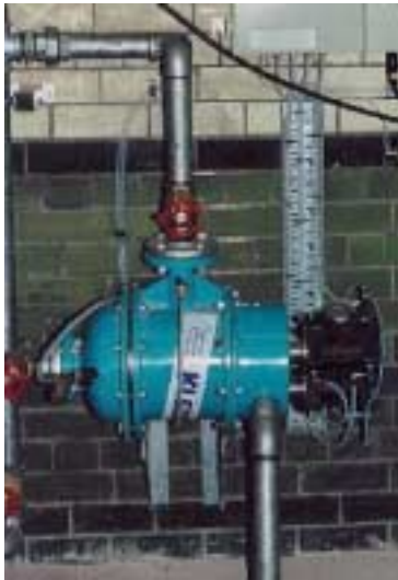
Municipal WTW UK 24 m 3 /hr River Water Pump Gland Seal Cooling
