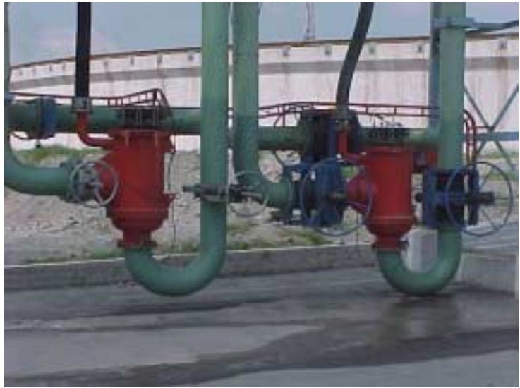
Platinum Mine South Africa 650 m 3 /hr each Protection of Pump Gland Seal Cooling and Instrumentation
